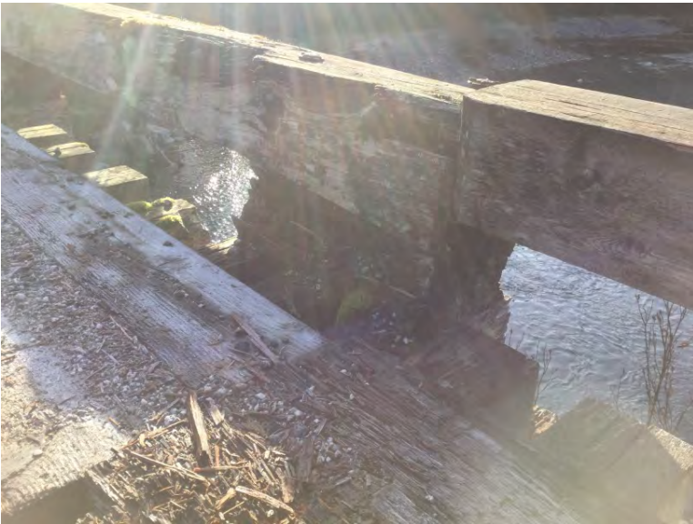
Guardrail condition poor
