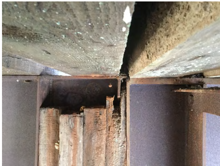
Upstream left span girder 10mm lower than right span girder
