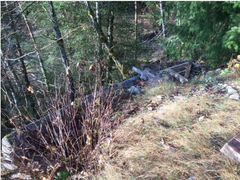
Downstream right bank barriers over bank
