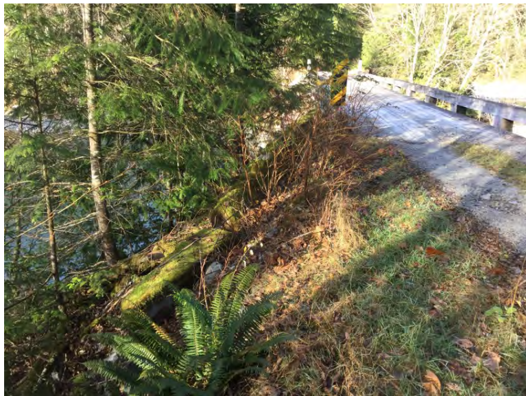
Downstream left bank barriers failing
