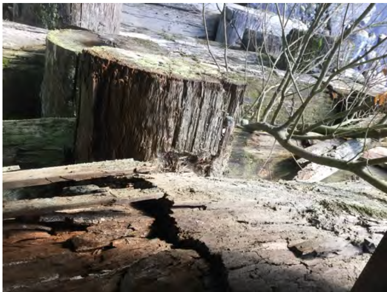
Vertical crack in top face log of left face of Pier
