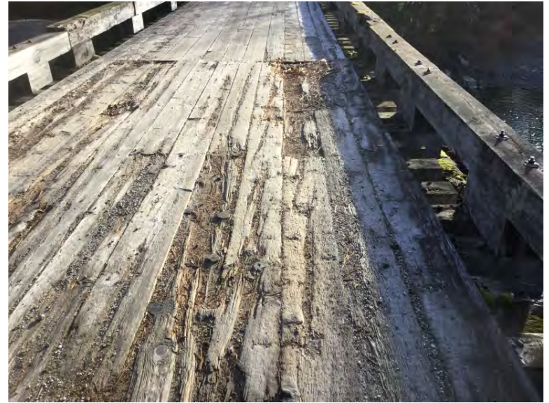
Plank condition on right span
