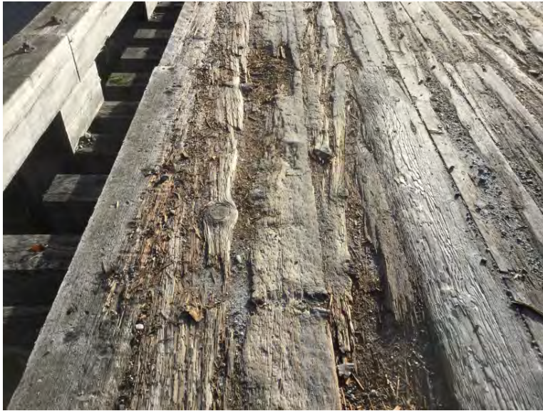
Plank condition on right span
