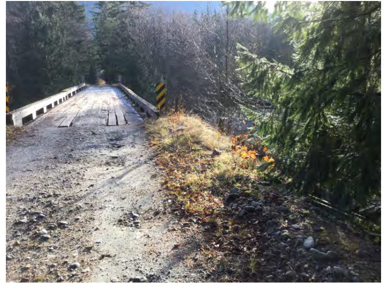
Downstream right bank barriers missing
