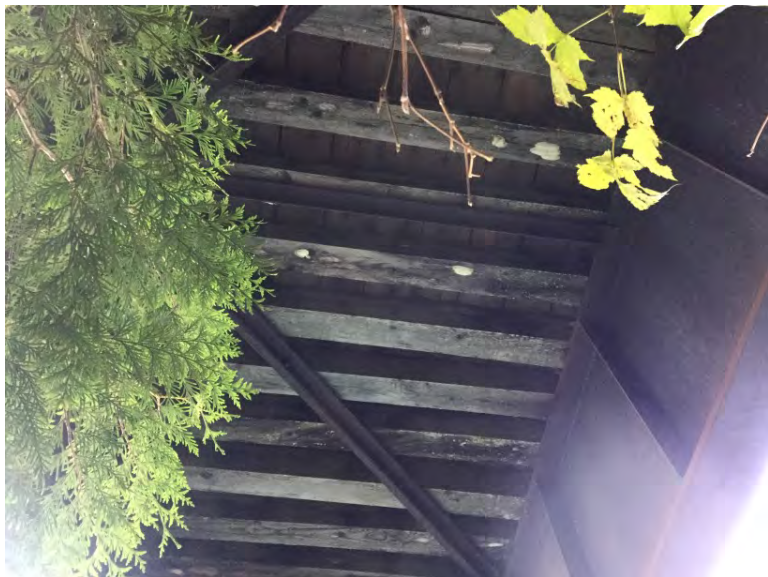
Left span tie condition
