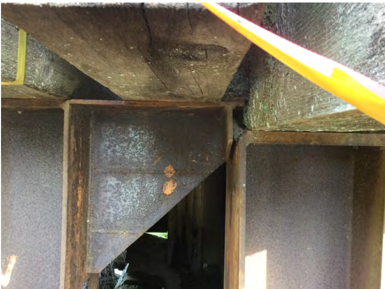
Downstream left span girder 63mm lower than right span girder
