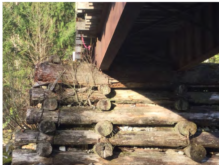
Top face log on left side of pier cracked through and girder settling
